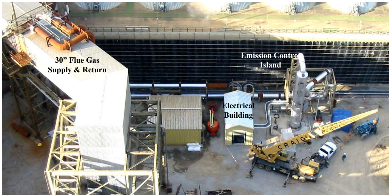
FIGURE 1: AIRBORNE DEMONSTRATION ABSORBER, EMISSION CONTROL ISLAND AND ELECTRICAL BUILDING
