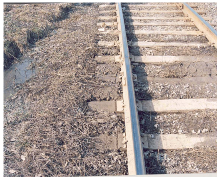
Figure 1. Contaminated ballast and track pumping
