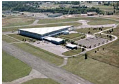
This aerial view of Rockcliffe's lower level shows the start of demolition of the hangars formerly occupied by the Museum (upper right). The Photographic Establishment "White House" (upper left) was torn down after the new National Aviation Museum opened in 1988. (National Aviation Museum 22032)
