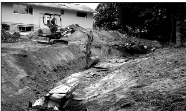
The stream had been lined with metal frames and topped with sheet metal, which was then covered over with fill.
