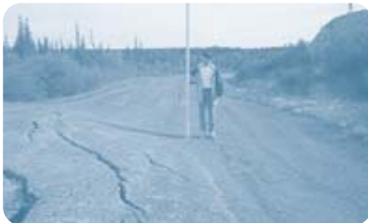
Tension cracks caused by slumping Ingraham Trail, NWT
