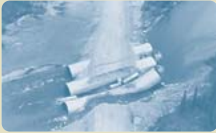
Washout on the South Canal Road
