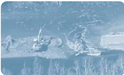
Wash-out, Yellowknife Highway 3, NWT
