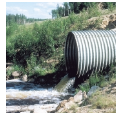
Poorly installed culverts are barriers to fish passage.
