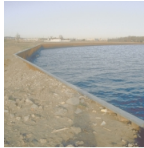
Vertical retaining walls provide little fish habitat.
