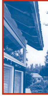
Open eaves, vents not screened (6 pts)
