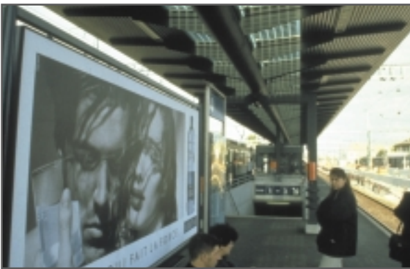
PV modules installed on the platform canopy at Morges railway station, Switzerland. The structure consists of a horizontal tube with a roof, glazed on both sides to let daylight through to the central part of the platform. (© EPFL-LESO)
