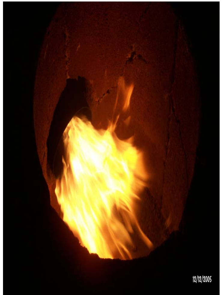
Typical #2 Fuel Oil Flame
