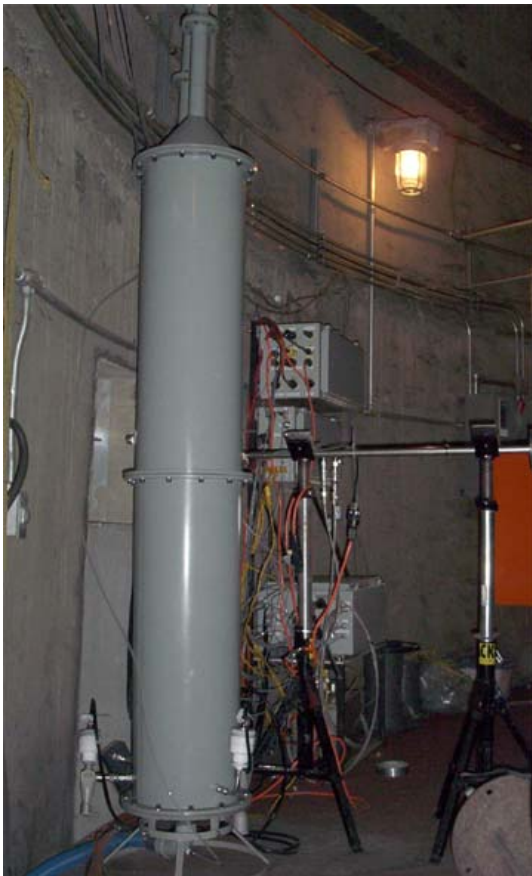
CETC-3 sampling system located inside utility stack
