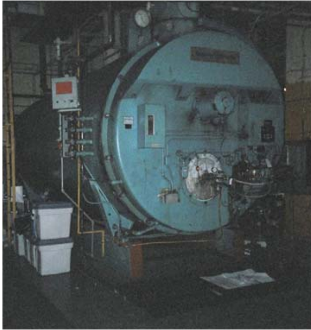
Residual fuel oil-fired industrial boiler
