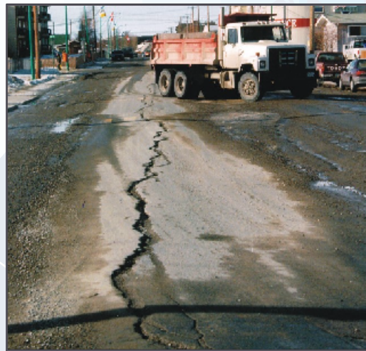
Crack developed in pavement due to frost heave in road foundation.
