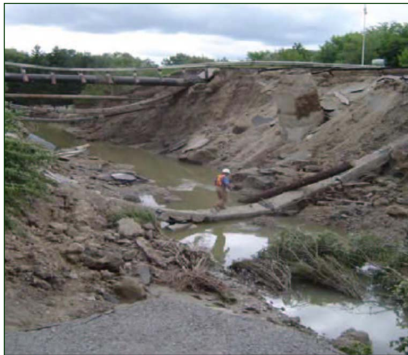
Figure 14: After a Severe Storm Event (August 2005): Eroded Culverts and Road, Finch Avenue: Toronto (D. Haley)
