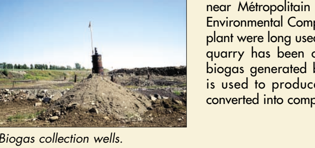
Biogas collection wells.
