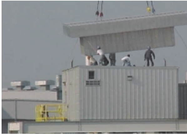
One of the 13 Big Foot air-heating units is delivered and installed on the roof of Ford's Oakville Assembly Plant.
