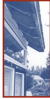
Open eaves, vents not screened (6 pts)
