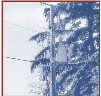
Contact utility companies for clearing of vegetation under overhead electrical installations.
