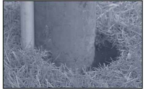
Faulty annular seal.
