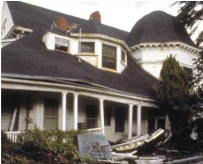
This turn-of-the-century wooden residence sustained major damage when it moved off its foundation during an earthquake.
