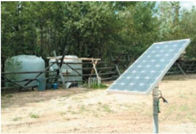
Irrigation water delivery system at the Takhini demonstration site.
