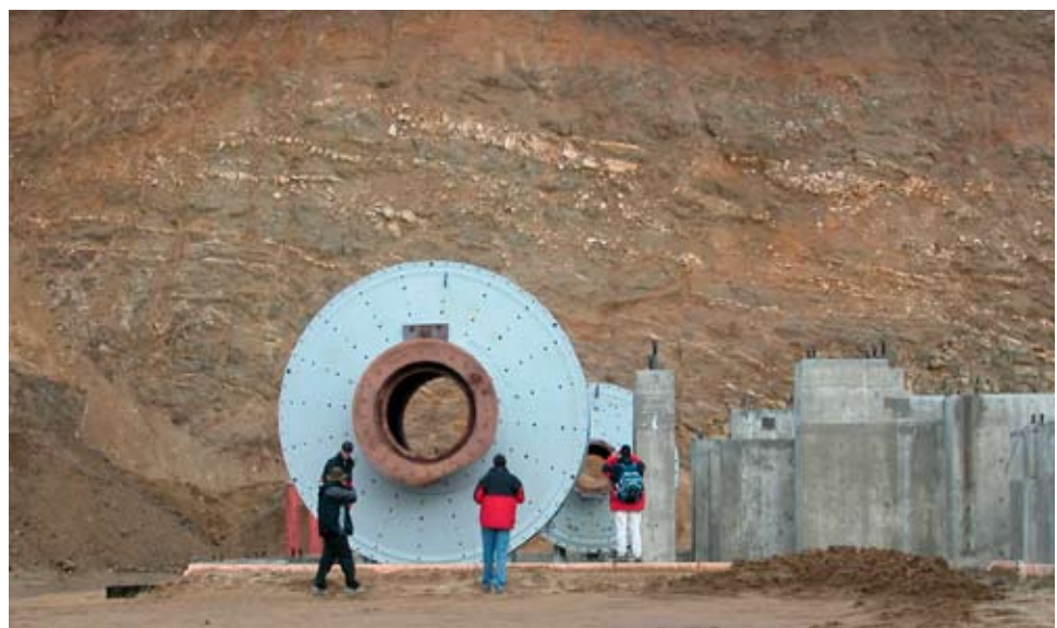
Figure 9. Semi-autogenous grinding mill, ball mill and mill footings at the Minto mine property.
