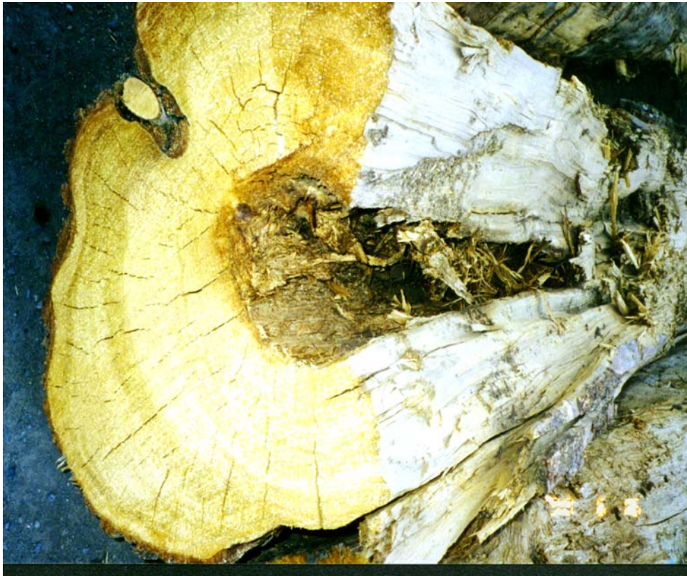
Figure 4.3 Butt rot with missing wood, showing how butt rot runs as a cone.
