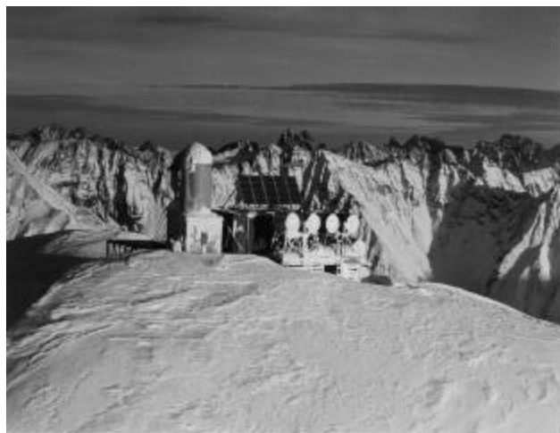
Figure 1. NorthwestTel Solar PV-Diesel Powered Microwave Radio Repeater
