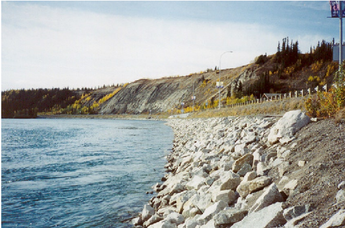
Plate 5. 'Granite' Rubble Used to Construct Breakwater along the Yukon River, Whitehorse, Yukon Pla5
