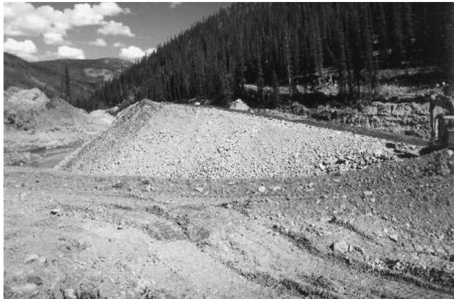
An example of a coarse pile bladed to an optimum grade of less than 2:1. Fine soils bladed into surface.
