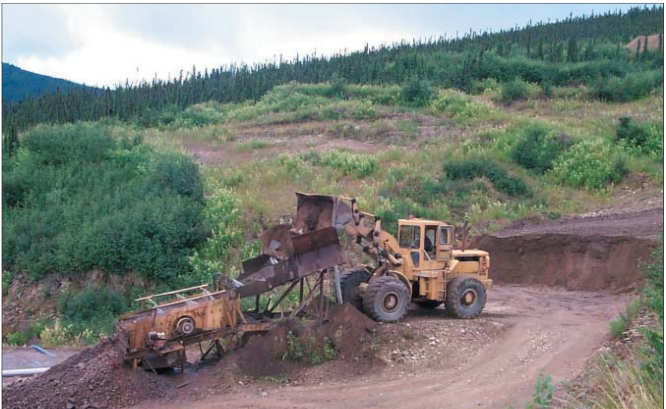
View of Jerry Bryde's shaker deck and sluice run set up in the mining cut on 7 Pup.
