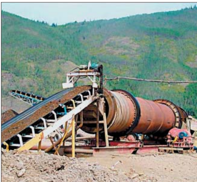
Tamarack's sluice plant on Indian River.
