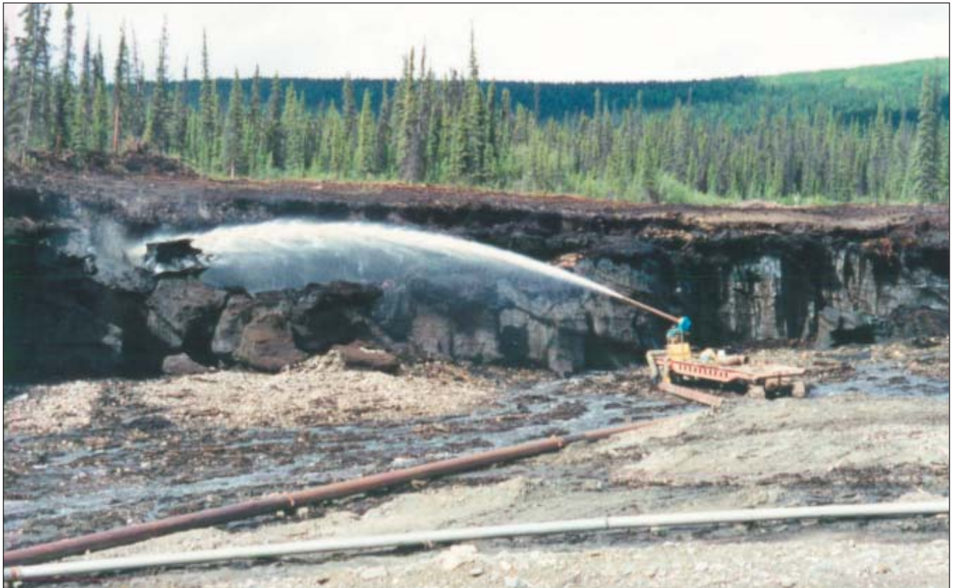
The automated hydraulic monitor used at Laskey Pup on Gold Run Creek by Ray Lizotte and Brent Construction.
