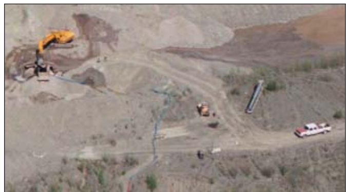
Sluicing on the left limit bench of Glacier Creek in 1998 under Erich Rauguth's water use licence.
