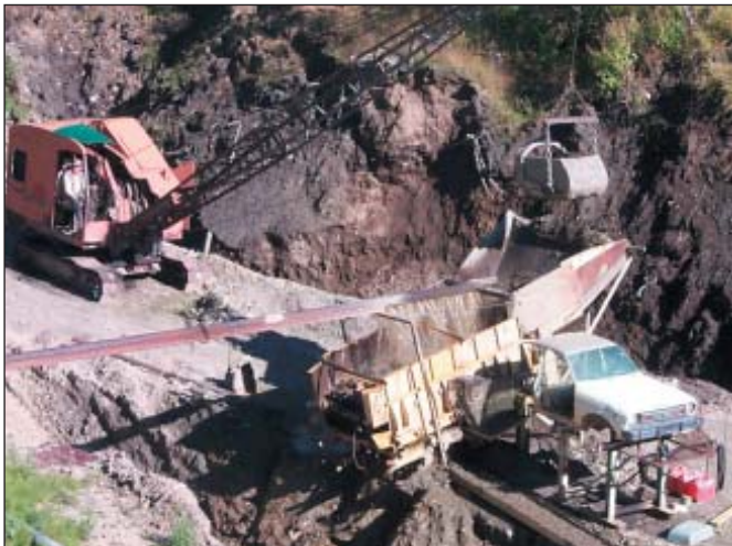
Close-up view of Alf Roberts using a drag line with ½ yard bucket, to dig pay gravel and feed the wash plant, in Homestake Gulch.
