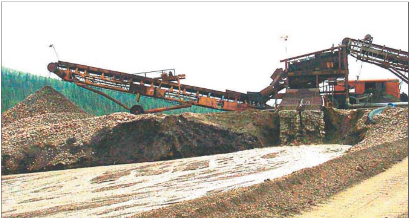
Lucky Lady's sluice plant on Sulphur Creek.
