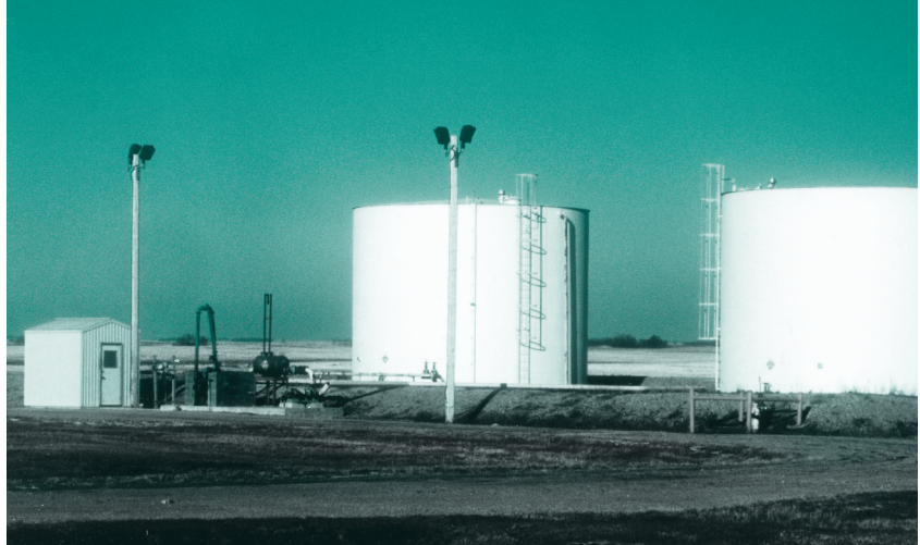
ETHANOL STORAGE TANK
