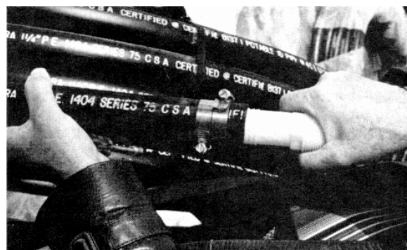
Stainless Steel Clamps in Opposite Direction.
