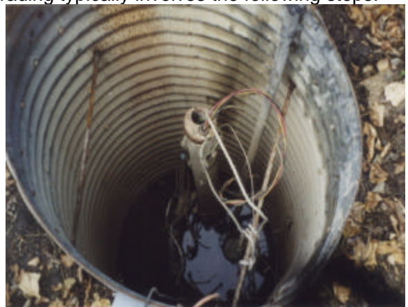
Well located in flooded well pit
