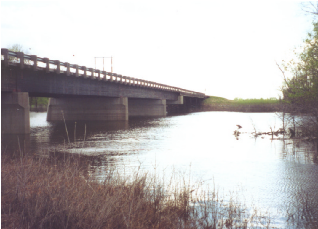
PHOTO E-9: RAT RIVER BRIDGE (ST. MARYS ROAD) NORTH ABUTMENT LOOKING SOUTH (D/S PIER NOSES) (May 17, 2001)
