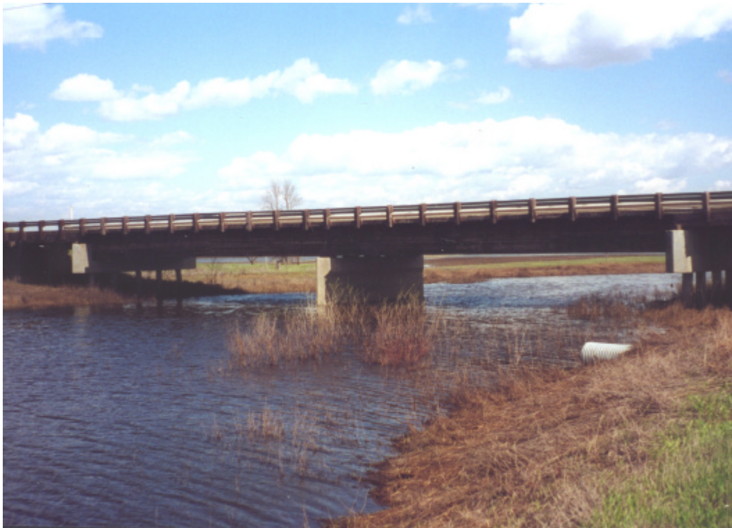
PHOTO E-8: APPROXIMATELY 30 M WEST OF ST. MARYS ROAD LOOKING EAST (U/S) AT BRIDGE OVER TOURAND CREEK (May 17, 2001)
