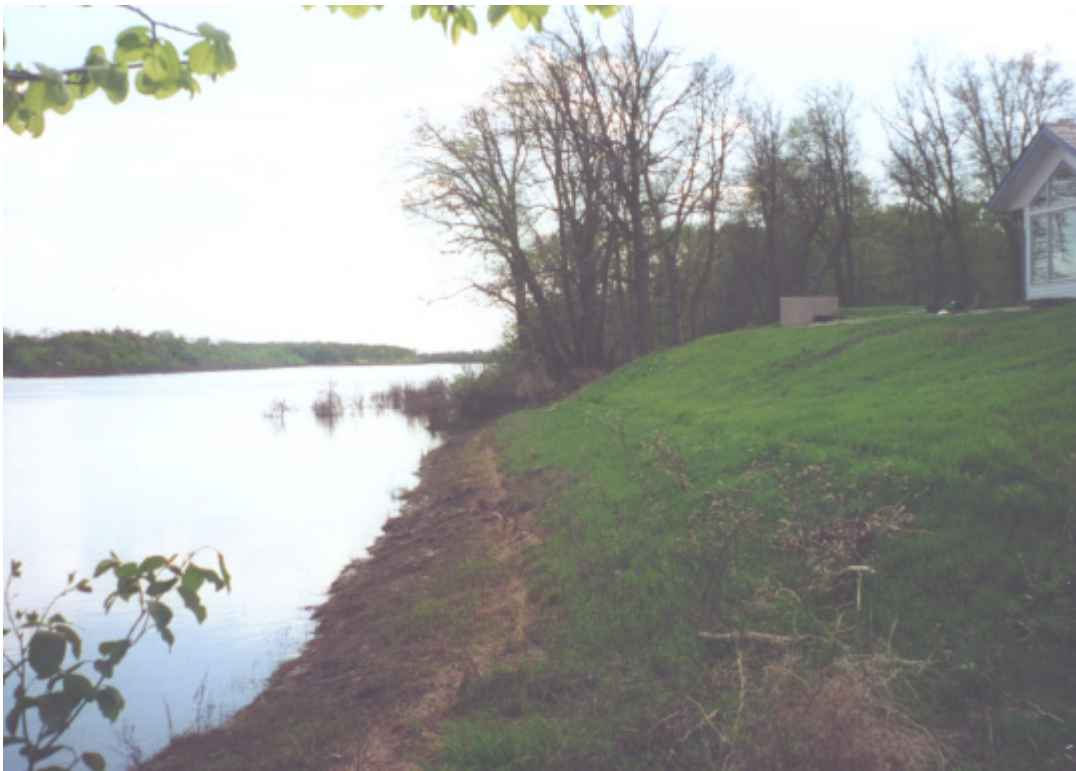
PHOTO E-6: EAST END CAMPEAU ROAD LOOKING SOUTH (WEST BANK) ALONG TOE OF RING DIKE (May 17, 2001)
