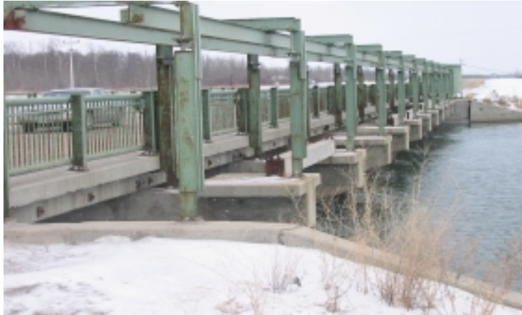
Above: Fairford River Water Control Structure
