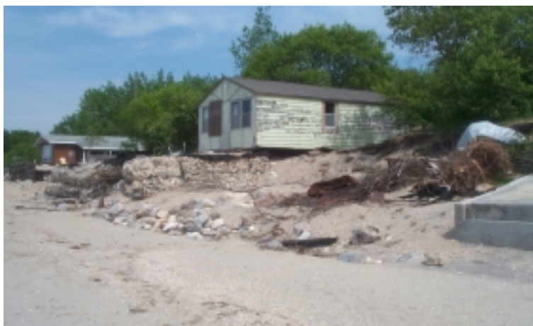
Above: Erosion damage to Lake Manitoba cottages.
