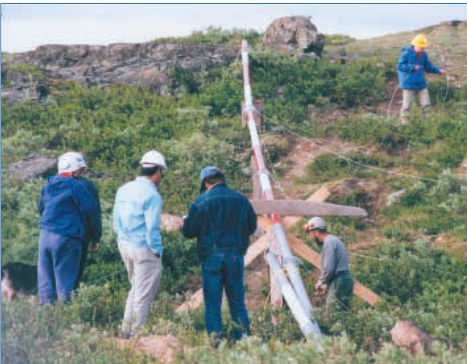
Craig family and crew on Haeckel Hill preparing tubular tower for lift, summer 1992.
