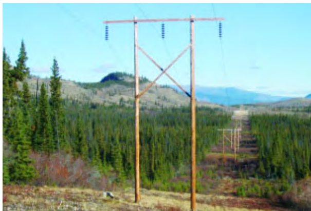
A 138 kV H-Frame transmission pole – Whitehorse-Aishihik-Faro Transmission Line
