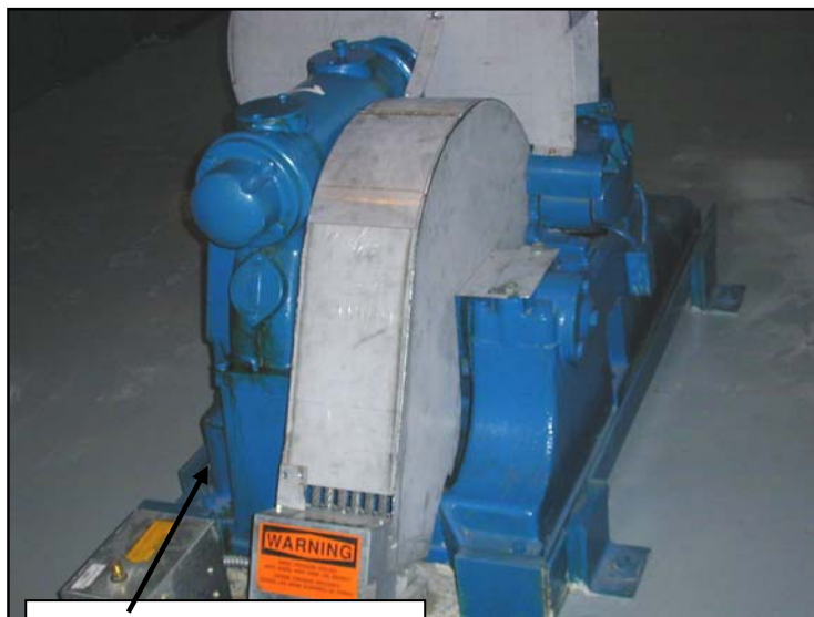
Fixed guard on sheaves Unguarded equipment
