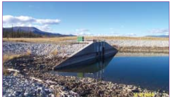
Flow control structure from lagoons.
