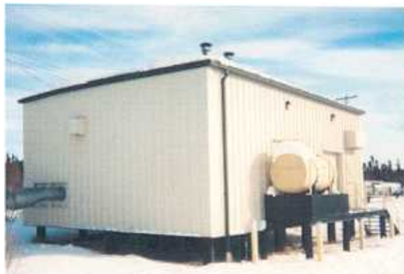
A UTILIDOR PUMPING STATION IN INUVIK.
