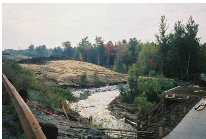
Figure 9. Construction zone in the area of the box culvert and stream diversion channel. A temporary berm was constructed to contain and divert runoff from the new section of highway away from the channel. The area down-gradient of the berm was stabilized with straw.
