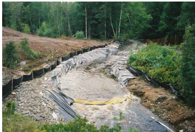
Figure 5b. The same section of the channel days after the same event. Note the displacement of the channel liner along a section of the east bank and stream channel at lower riffle.
