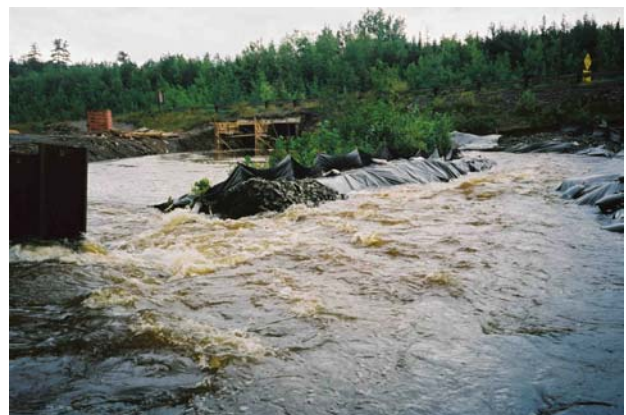
Figure 4. Washout of diversion trench sidewall during September 11-12 rain event. View is looking downstream.
