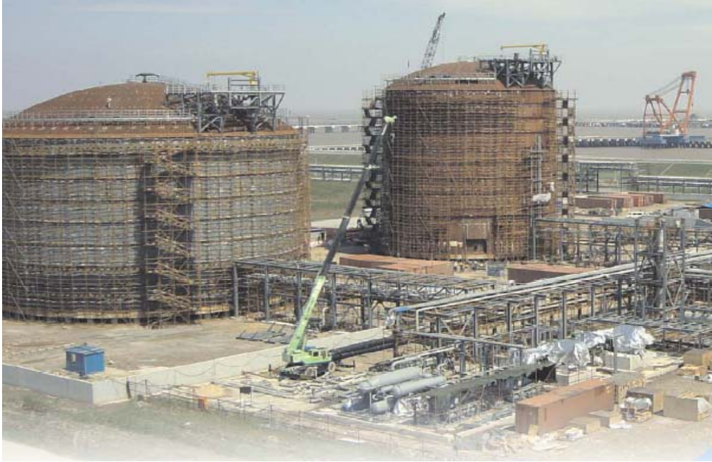
FIGURE 2.5-18 Typical Ethylene and Propylene Storage Tank
