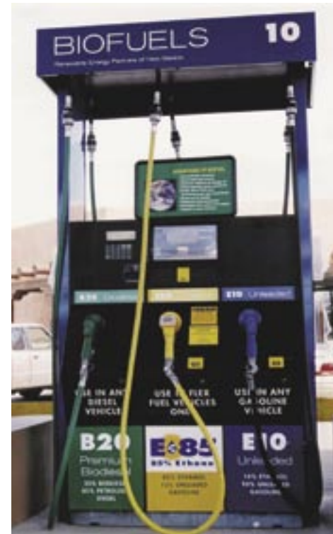
Multi renewable fueling station
