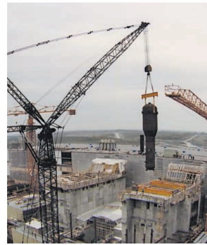
A steam generator can be installed in one or two days, using a VHL crane to lift equipment through the top of the reactor building, as compared with two weeks for the traditional horizontal-access method.
