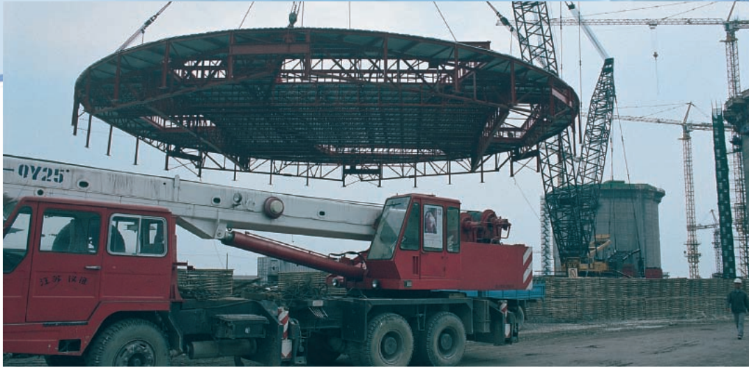
Preparing for open-top construction, a temporary roof is installed on Unit 2 of the Qinshan Phase III CANDU project in China.
