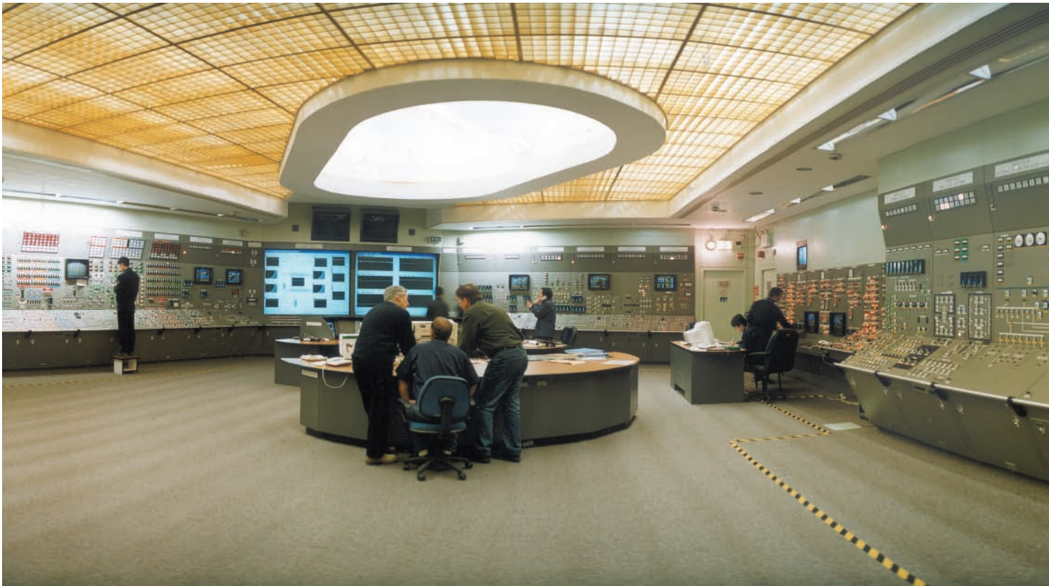
Qinshan Phase III Unit 1 control room
