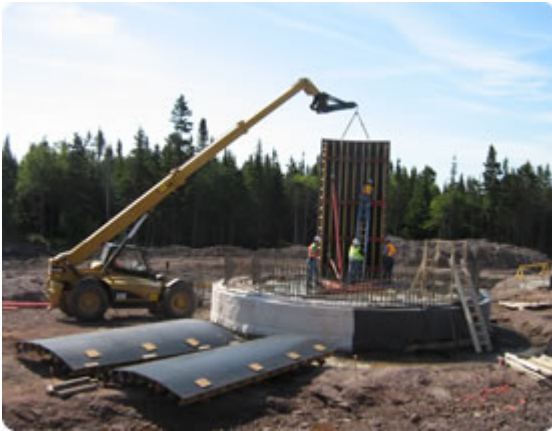
Erecting circular tie-less formwork for the retube canister walls of the waste management facility.
