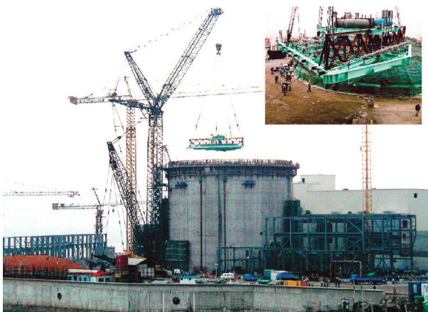
Use of open top construction method reduced installation schedule of dousing system from 6 months to 5 days
