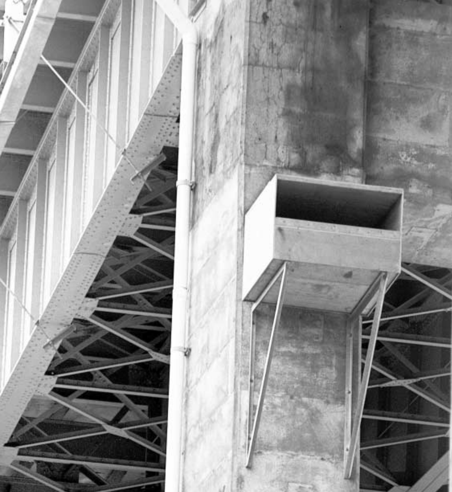
Falcon nests such as this one located underneath the Honoré Mercier Bridge, help prevent this protected species from nesting directly on the structures, potentially delaying upcoming maintenance activities.
