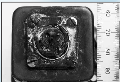
Relay end of the connector showing the damage to the three phase pins and the melted connector case.
