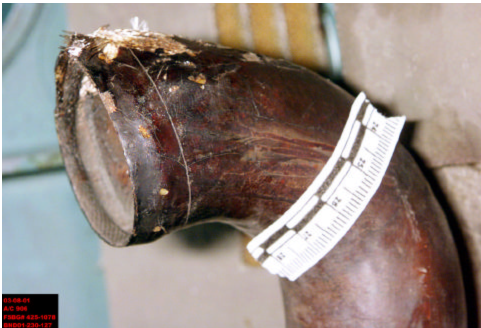
Photo 4: Fibreglass duct, found disconnected and chaffed at the turbine attachment point.
