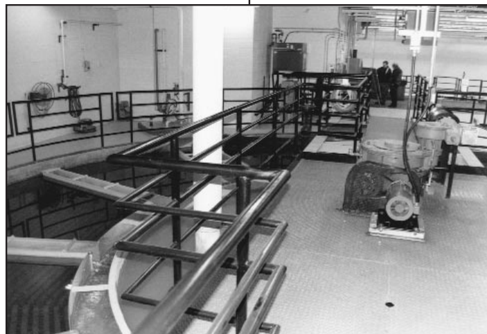
SOLIDS CONTACT UPFLOW CLARIFIER
