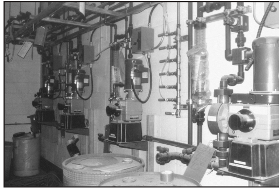
CLEAN IN PLACE PUMPS
