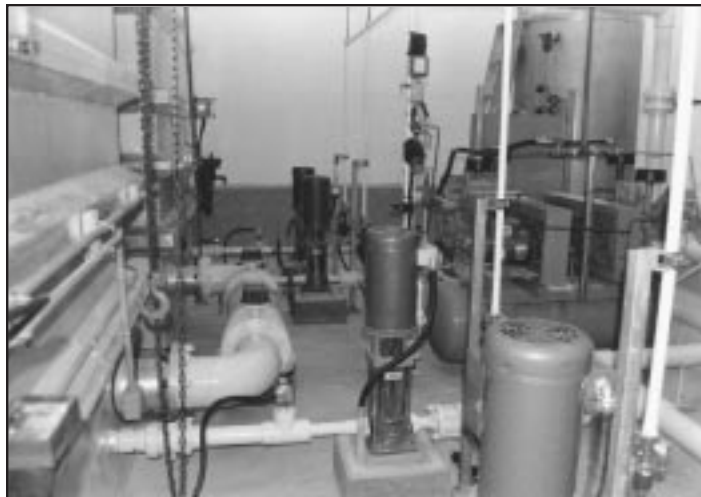
CONTROLS AND PUMPING
