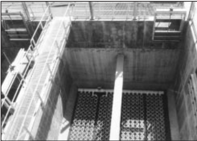
DIFFUSER SYSTEM ACTIVATED SLUDGE TANK
